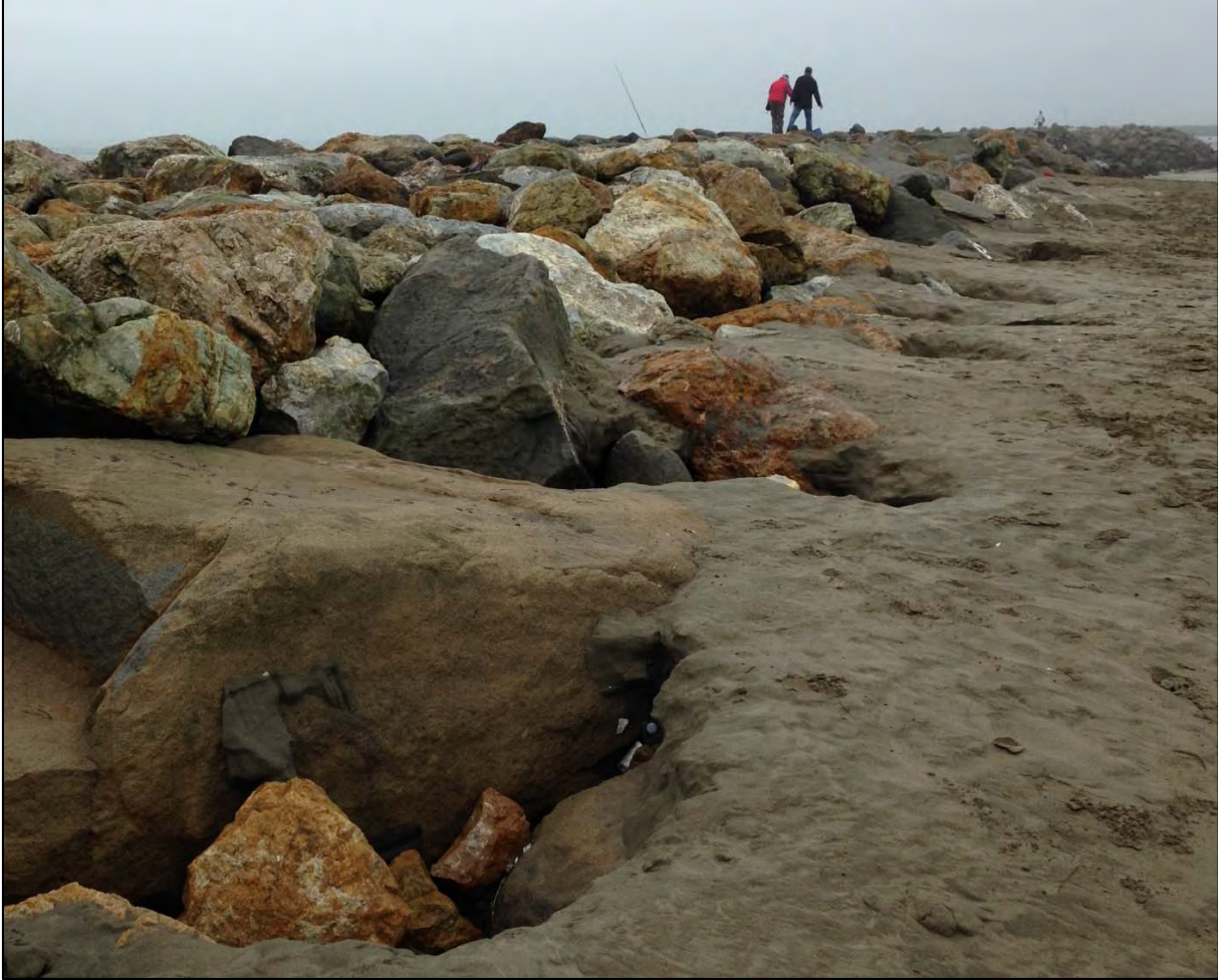
Figure 49. Photograph showing areas of scour due to surging along the harbor side of the east breakwater (Source: James Zoulas)
